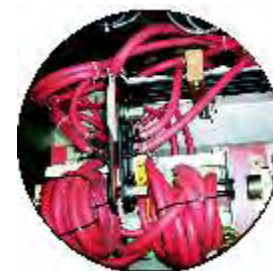
INDUCTION COIL CHAMBER
